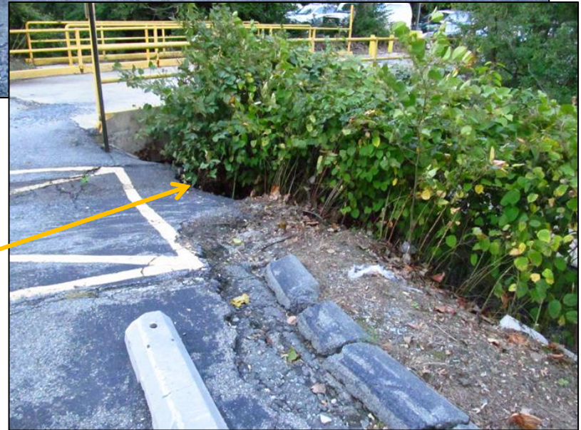
Edge of parking lot eroding and falling into creek.
