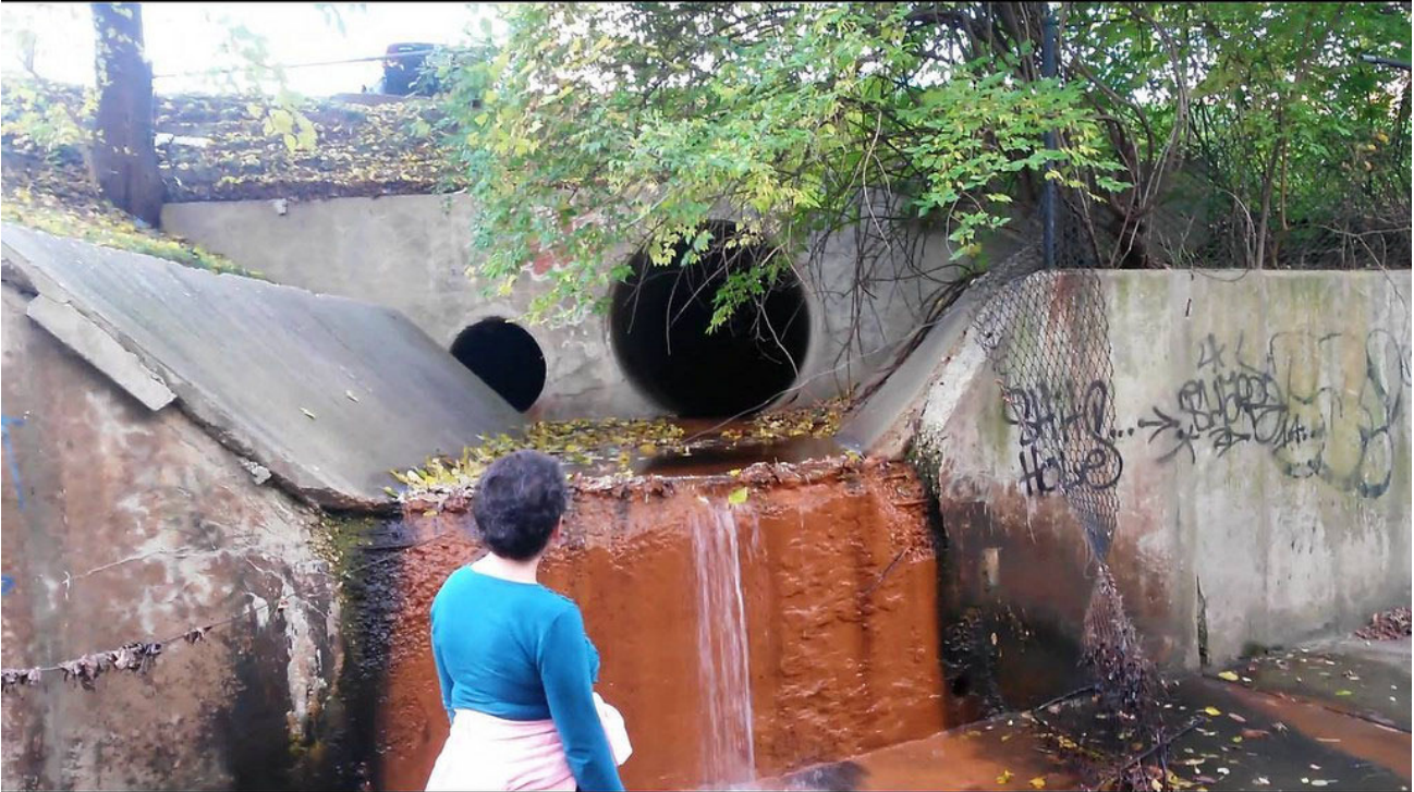
Figure 1: Kenwood Tributary outlet to the Willett Branch at River Road, adjacent to the Westwood Center II parking lot
